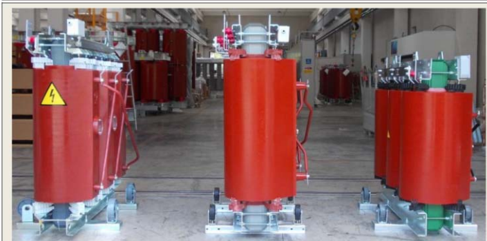
TRANSFORMER A TESAR TRANSFORMER B
