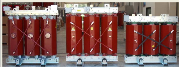
TRANSFORMER A TESAR TRANSFORMER B
